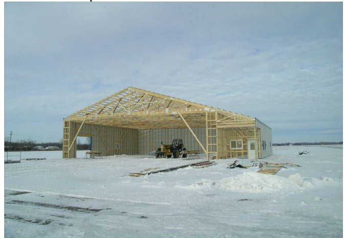
Here's Curt's hangar on Sunday, December 9 th . By now it is nearly finished.
