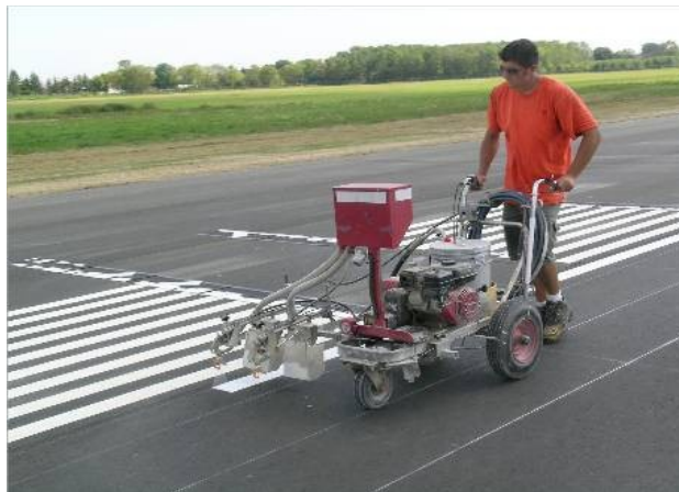
September 5 th . Two days until opening and the numbers are being painted on the runway.
